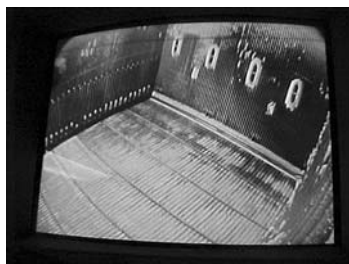
Internal view of the boiler in Maine prior to start-up, showing four new OFA openings on the right side wall. Jansen's design of few but large OFA nozzles facilitates deep air jet penetration and excellent OFA cross-sectional coverage, therefore greatly enhancing boiler performance.
