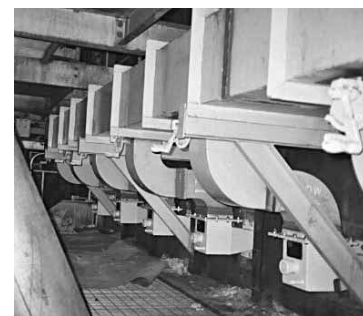
Five of six Jansen OFA nozzles are shown on the front wall of the No. 7 Power Boiler, including supply windbox, ducting, and supports.
