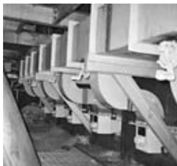
Five of six Jansen OFA nozzles are shown on the front wall of this biomass boiler, including supply windbox, ducting, and supports.
