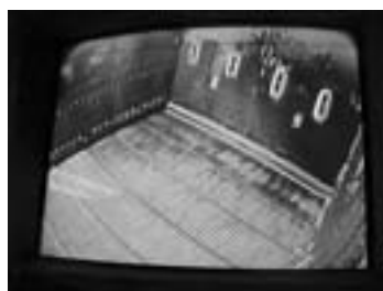
Internal view of a biomass boiler prior to start-up, showing four new OFA openings on the right side wall. Jansen's design of few but large OFA nozzles facilitates deep air jet penetration and excellent OFA cross-sectional coverage, therefore greatly enhancing boiler performance.
