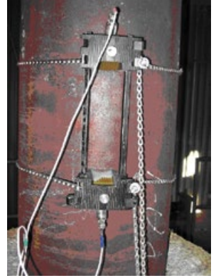
Jansen UFM instrumentation for measuring water velocities in main downcomer.
