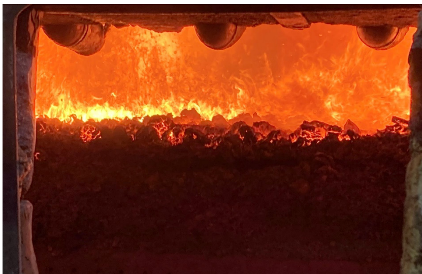
Combustion on a Coal-Heavy Grate
