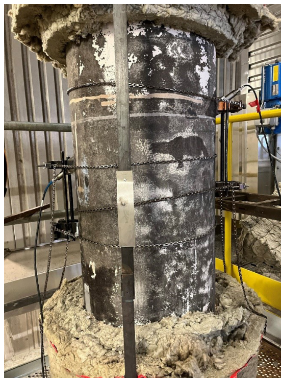
Water Flow Measuring Equipment on Boiler Downcomer
