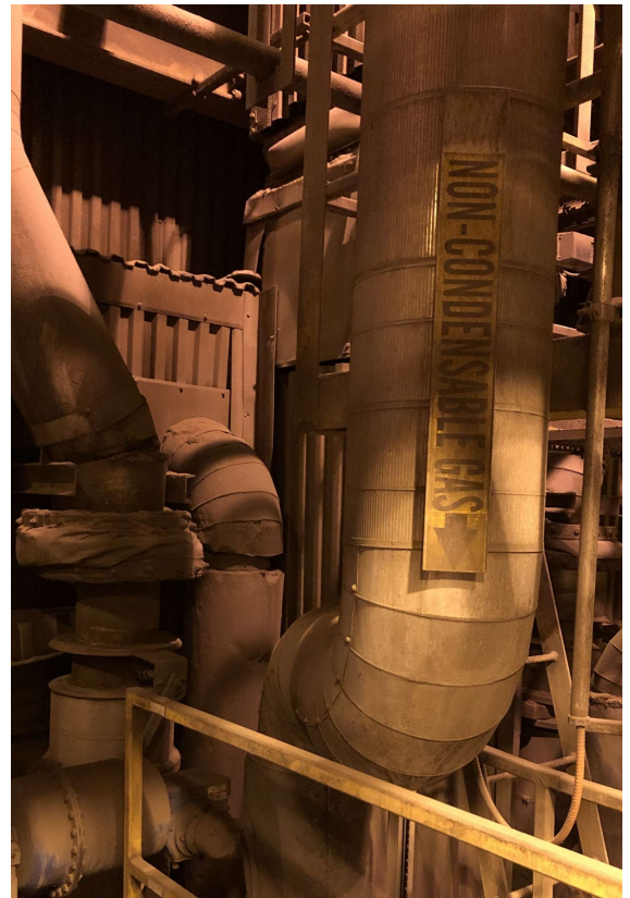
NCG Pipe Feeding Fluidized Bed Boiler
