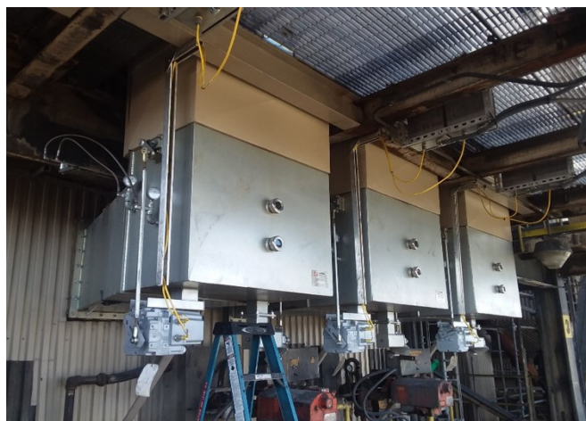
Jansen Overfire Air Nozzles on an RDF-fired Boiler
