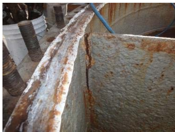
Failed Surface Condenser Baffle
